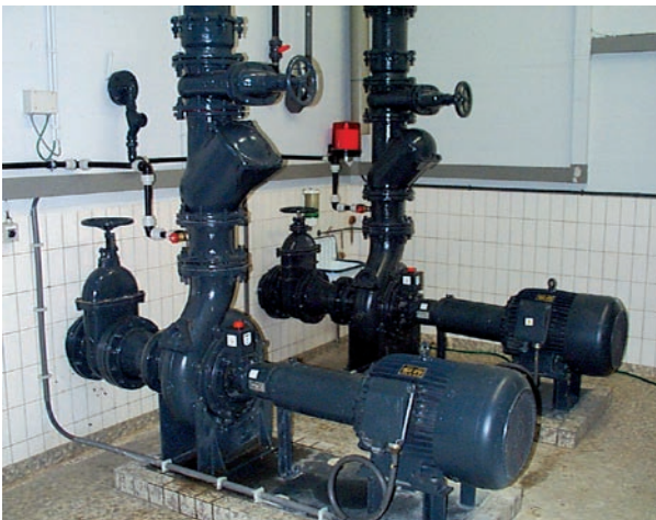
Flygt dry installed pumps, the ultimate solution for solids handling applications. Above two pumps managing the sewage system at Amsterdam airport "Schiphol".
